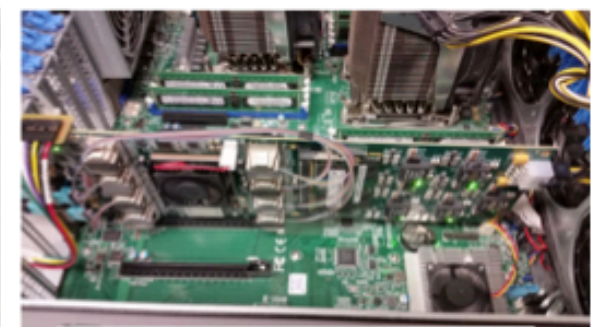
Installed in a Server
