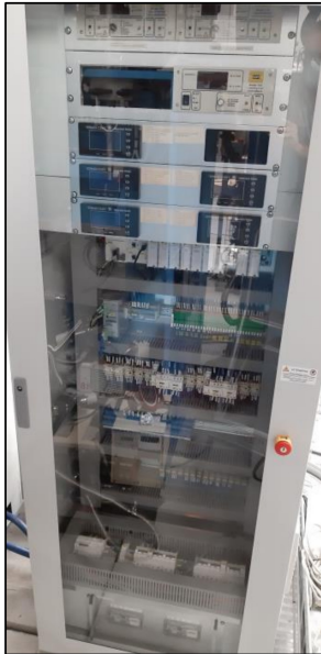
SRFQ electric board
