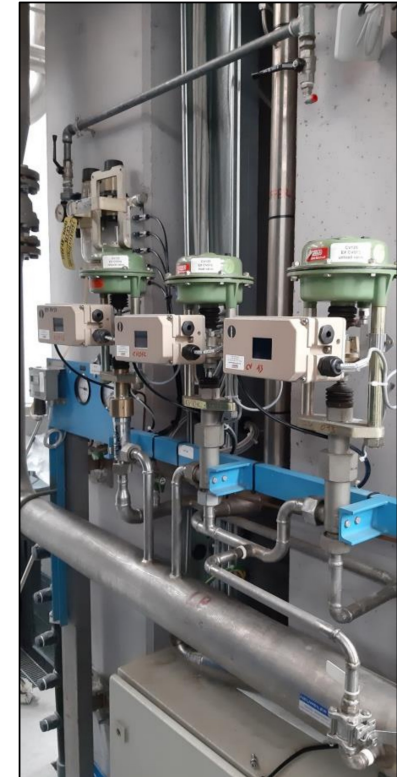
Gas control panel
