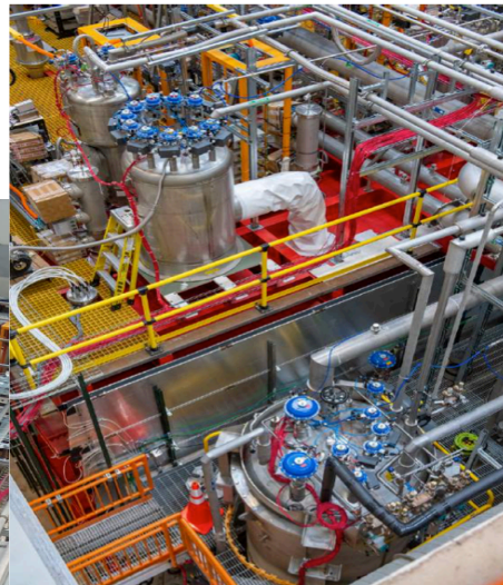
All cryogenic equipment installed/test ed (May 2019)
