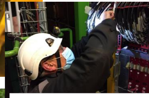
Muon electronics installation
