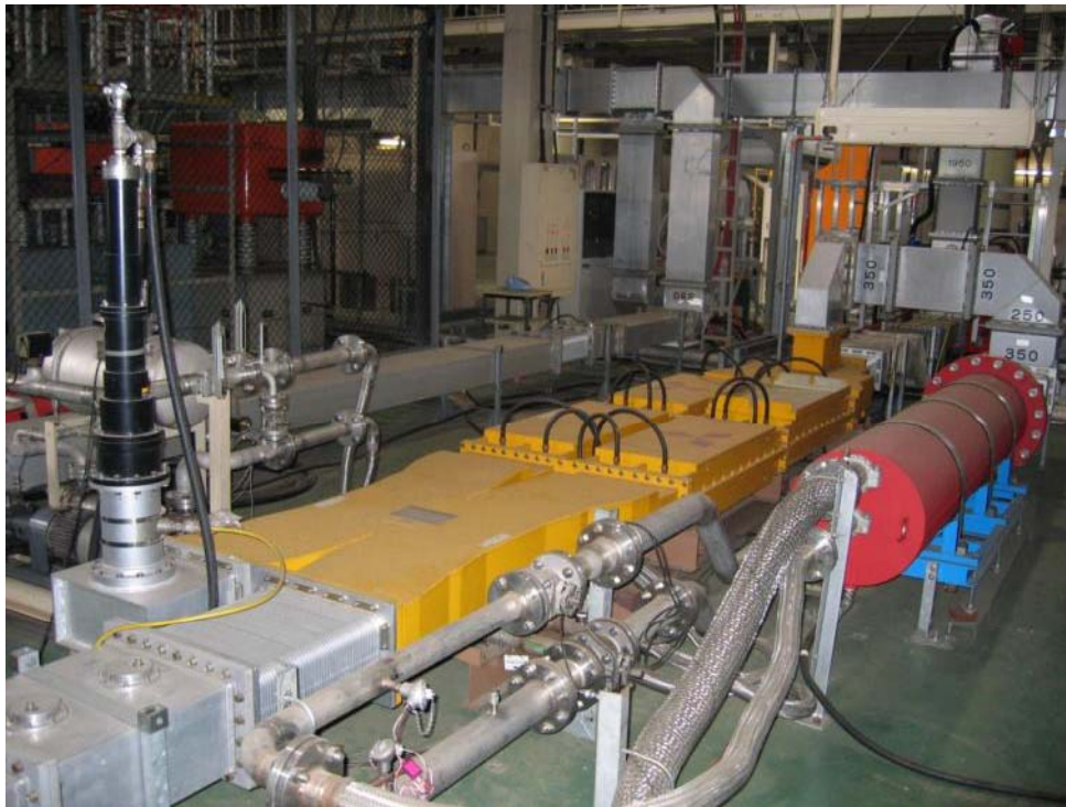
High power RF system
