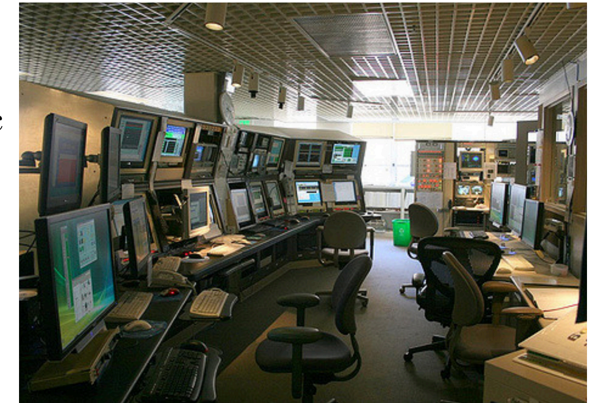
High level controls
