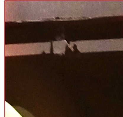
Broken HV lines
