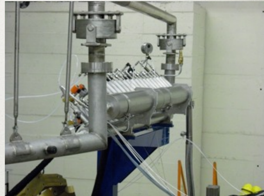
AUTOFILL HARDWARE MAINTENANCE
