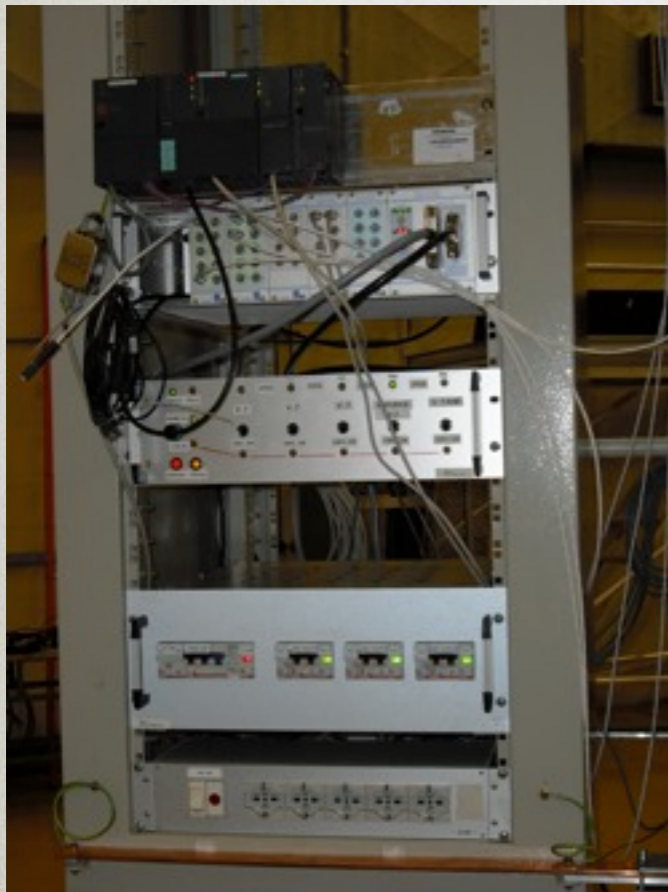
VALVE POWER SUPPLY AND CONTROL CRATE
