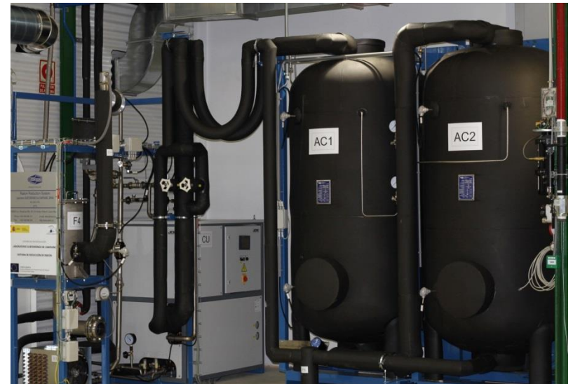
Chiller and charcoal filters, Hall A at LSC
