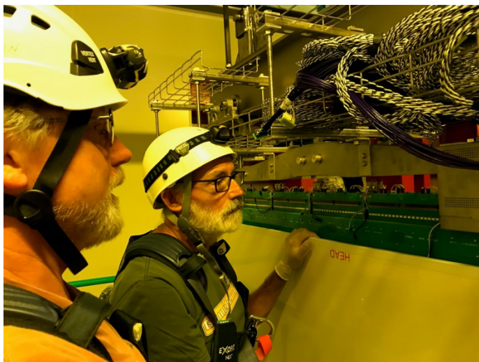
Cabling on cable tray
