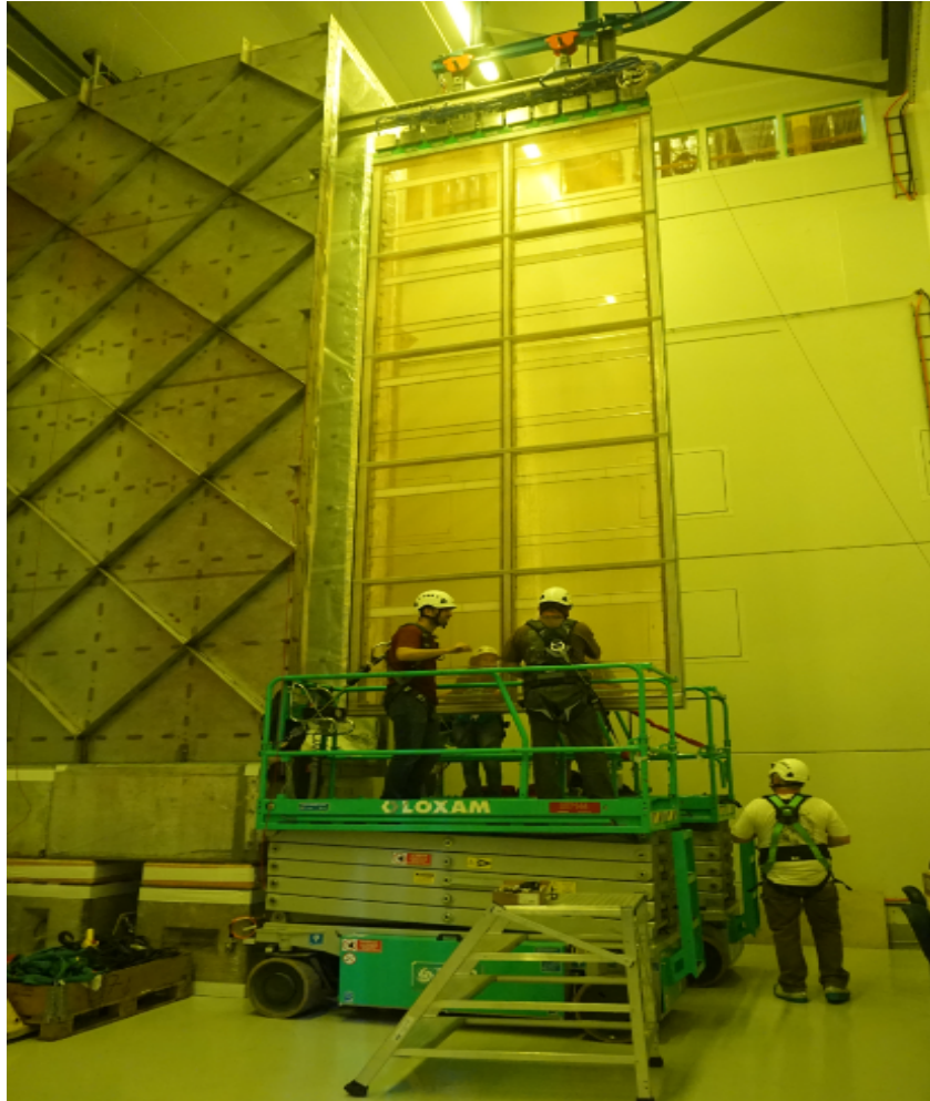
APA being moved into Cold Box
