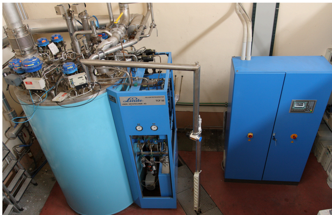
LINDE TCF 50 liquid He liquefaction/refrigeration plant
