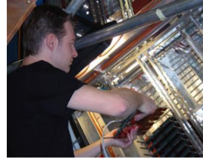
Install new FEC + test
