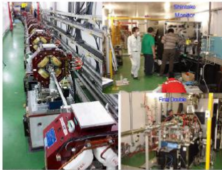
Fig. 4: ILC ATF2 beam line magnets
