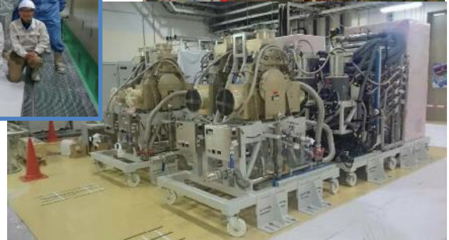
RF power system under completion
