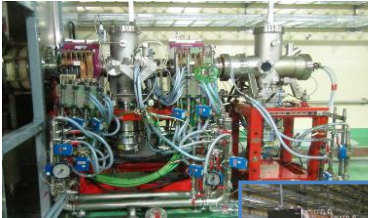
Injector under commissioning
