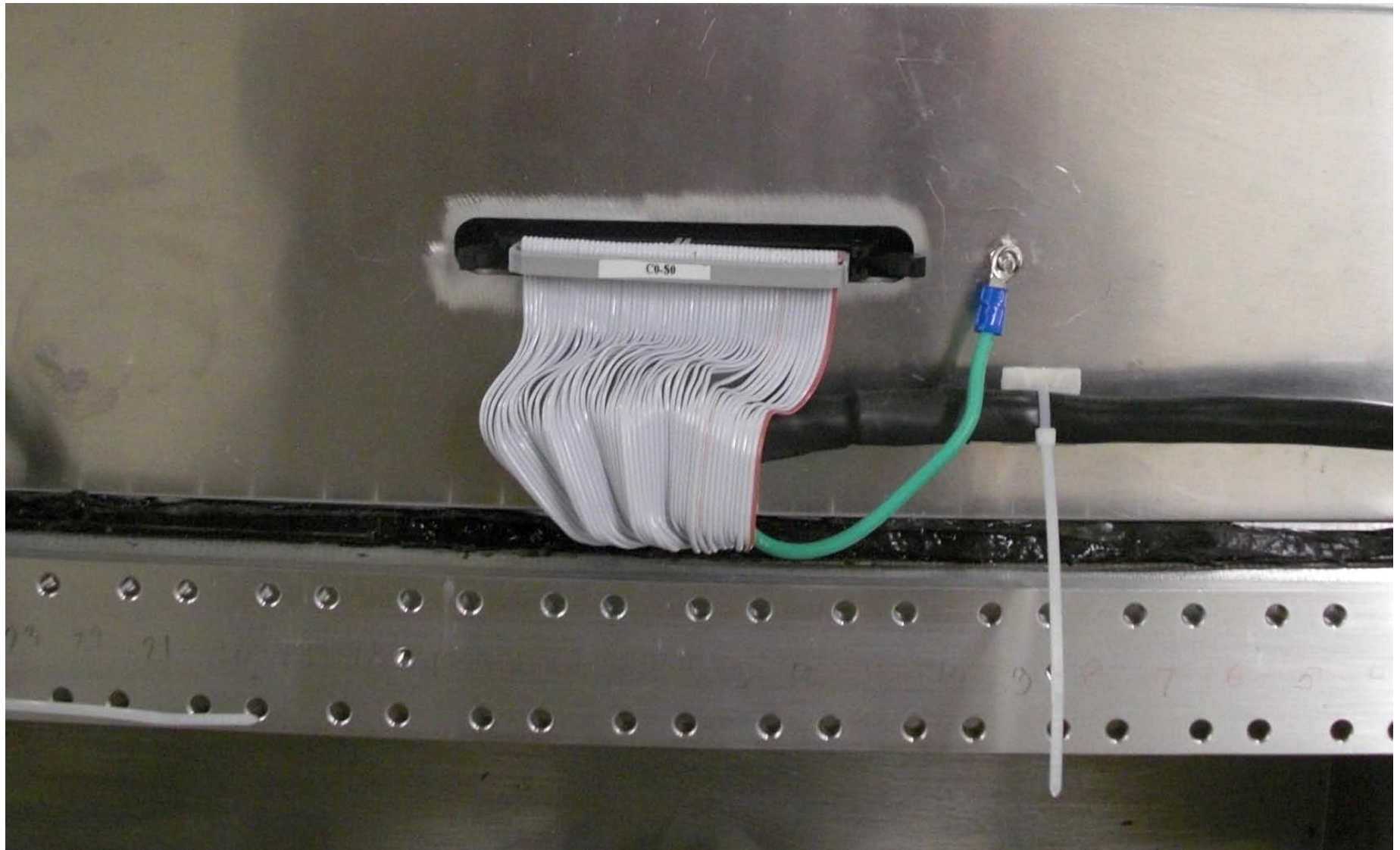
Cable and fiber installation in process – Final checkout = APD + PreAmp + cable + fiber bundle + 3mm fiber
