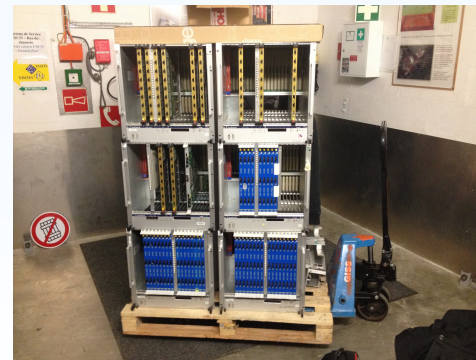
VME system ready for storage
