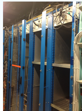
Empty Racks Cables in false floor
