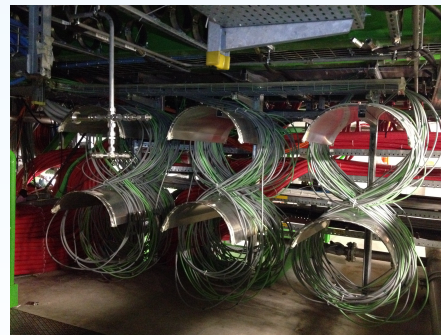
Slack storage in false floor
