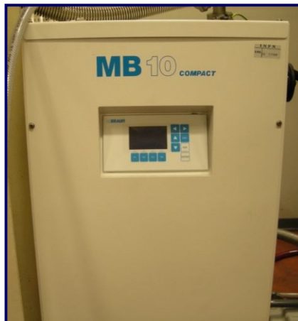
Recirculation system and gas purification
