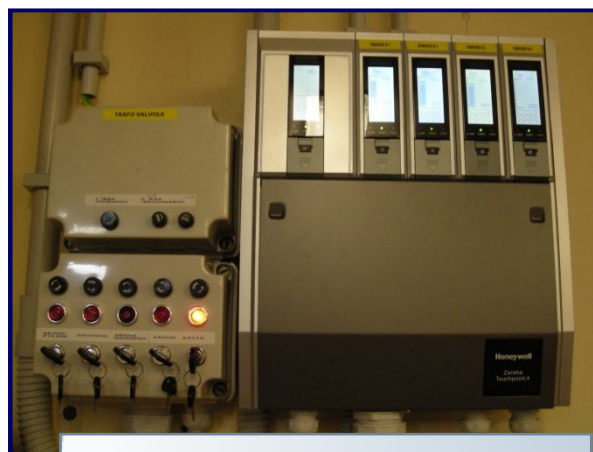
New gas distribution unit + O 2 sensors
