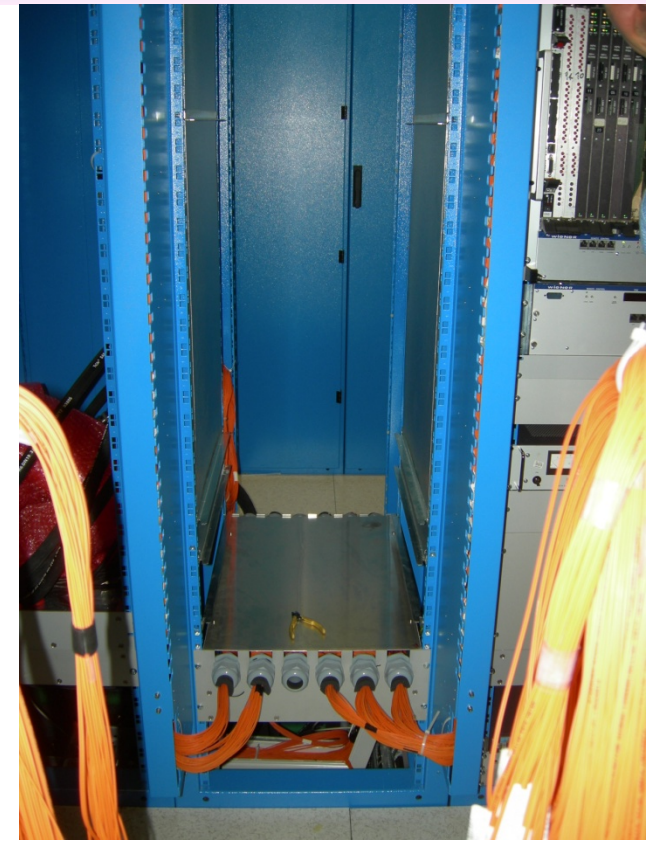
Both racks now equipped with the final ATCA shelves
