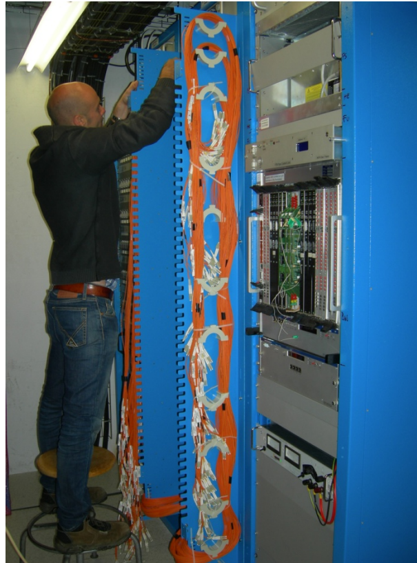
Fibers installed and fixed inside the fiber tray
