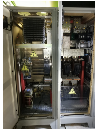
KLOE PS Dump resistor and contactors
