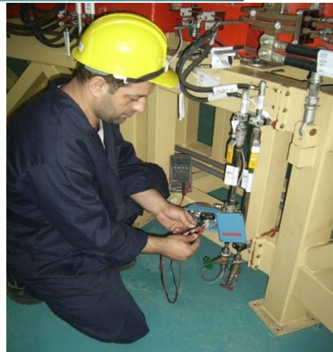
Flow Switch Test
