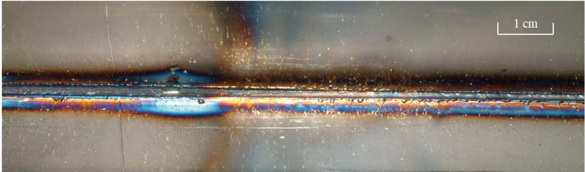
Figure 4. Damage observed on the inside of the vacuum chamber, on the beam impact side. A groove approximately 110 cm long due to removed material was clearly visible, starting at about 30 cm from the entrance.
